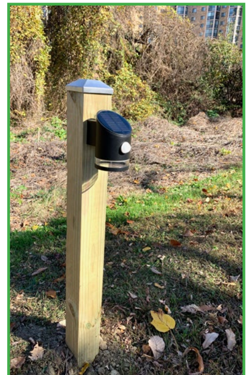
A 35-inch tall solar light on the Metro road
