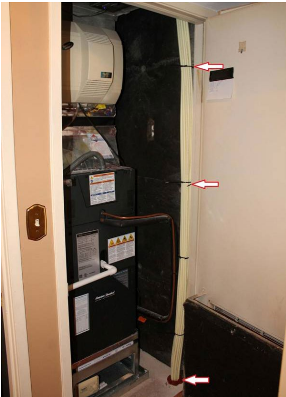
The Fios cables bundled with cable ties, Fios cables not shielded inside conduit or even PVC pipe.
