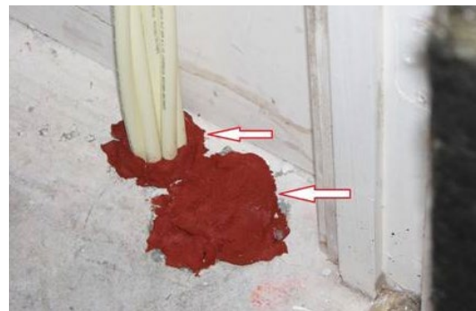
The drill team remediated their errors with the sealing compound. How permanent is this solution and is this level of performance the Montebello is paying for?
