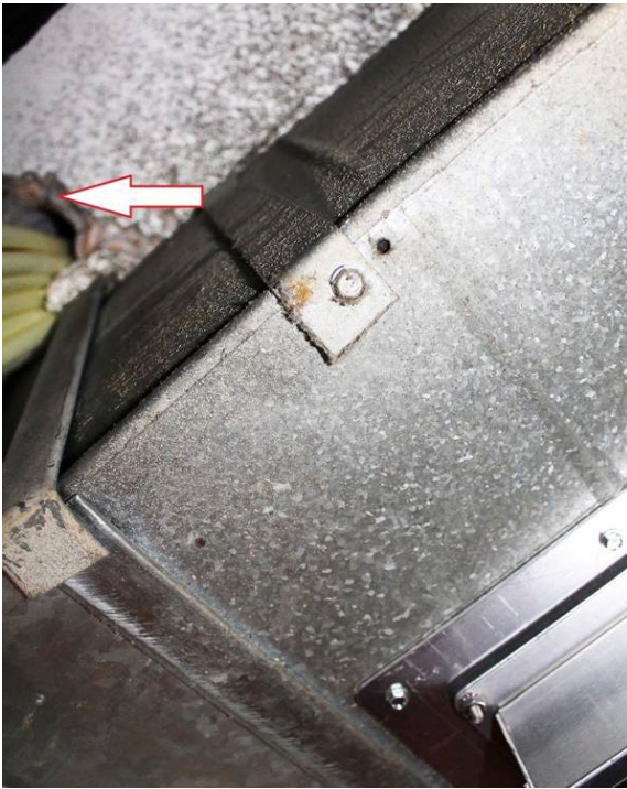
Fios cables enter HVAC closet via hole in ceiling. Note the jagged hole, no sealing around cables and no conduit pipe to protect cables.
