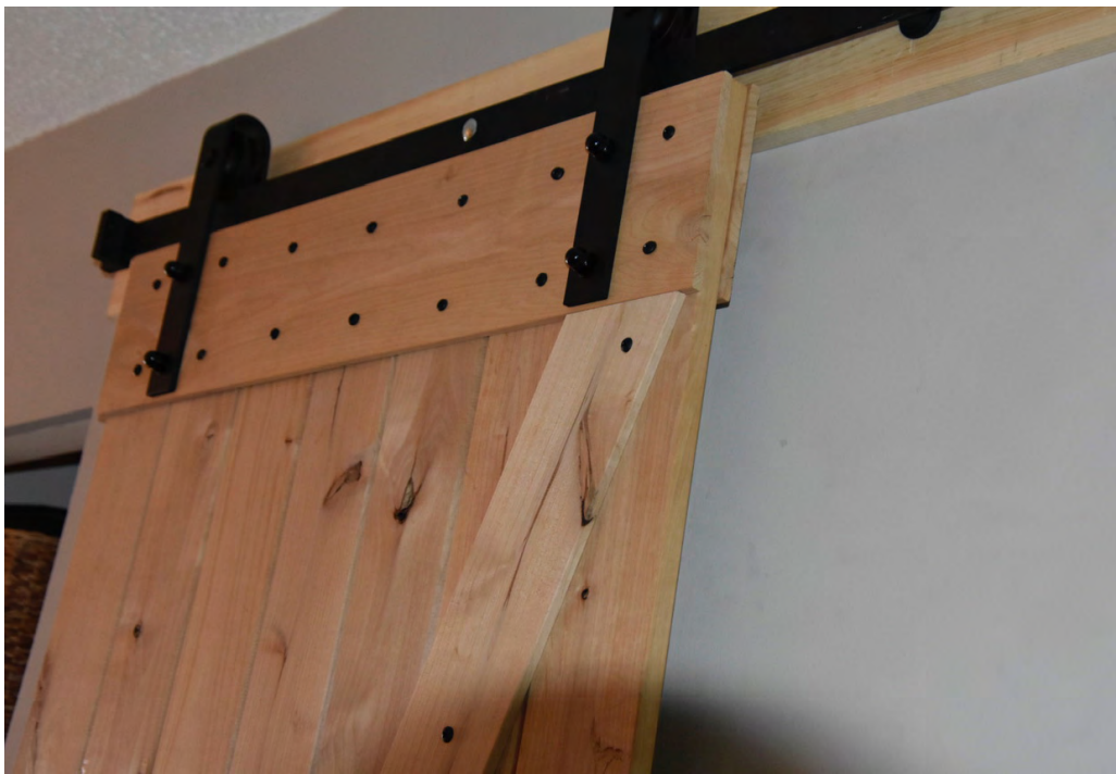
Mike Brownlee's new door closet project Building 2 balcony Photos by Linda Brownlee
